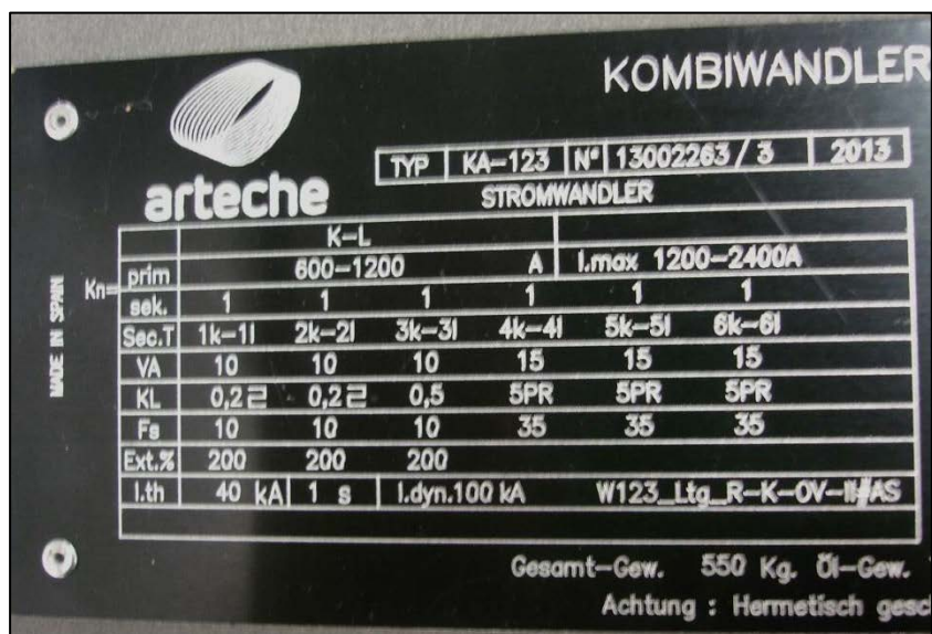
➤ Figure 1 – Arteche KA-123 Rating plate of current transformer.
